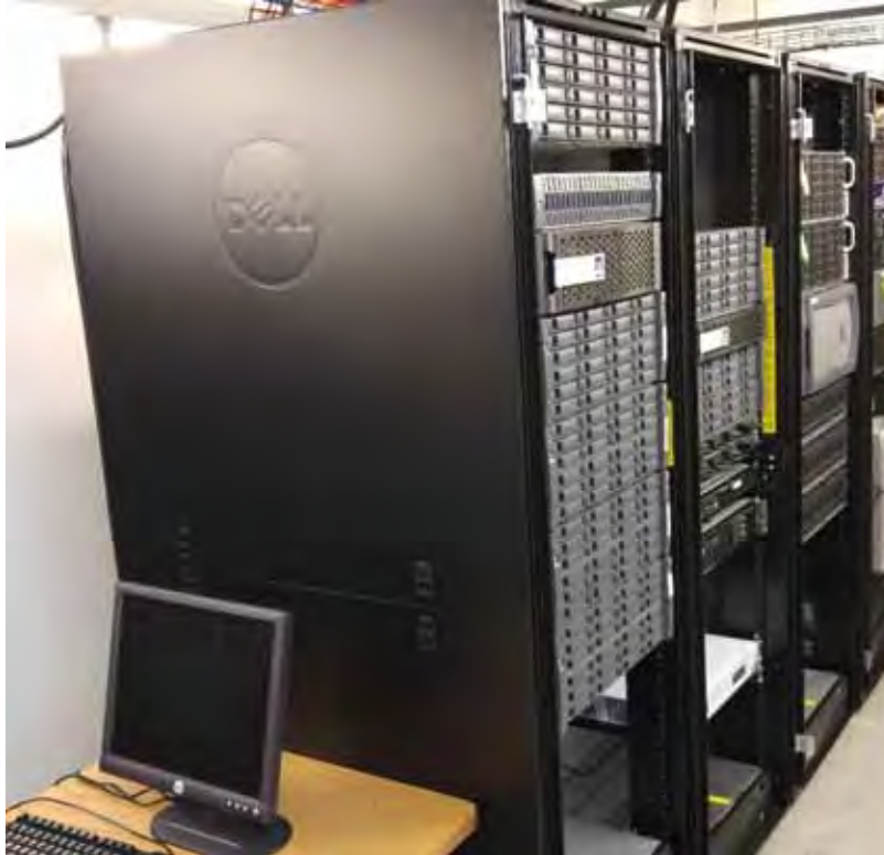
Figure I-7. Center SAN and NAS infrastructure in the primary server room.
