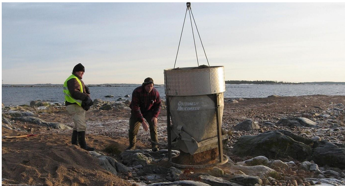
Figure 15. Stenarna 19/12 2007. Ulrik Lötberg and Per Nordkvist guide a barrel of gravel to the ground and empty its contents. Now the gravel must be quickly distributed before the next delivery. Photo by Uppsala county administrative board, Niina Salmén.
