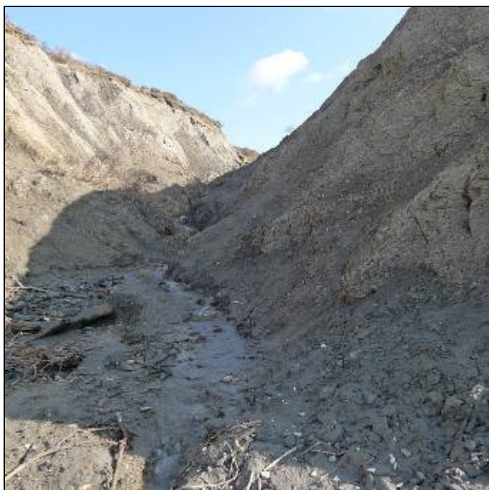
Plate 7. Actively eroding stream gully near Waypoint 710
