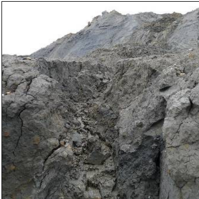
Plate 5. Small rivulet just above beach. Note the recent landslip above.
