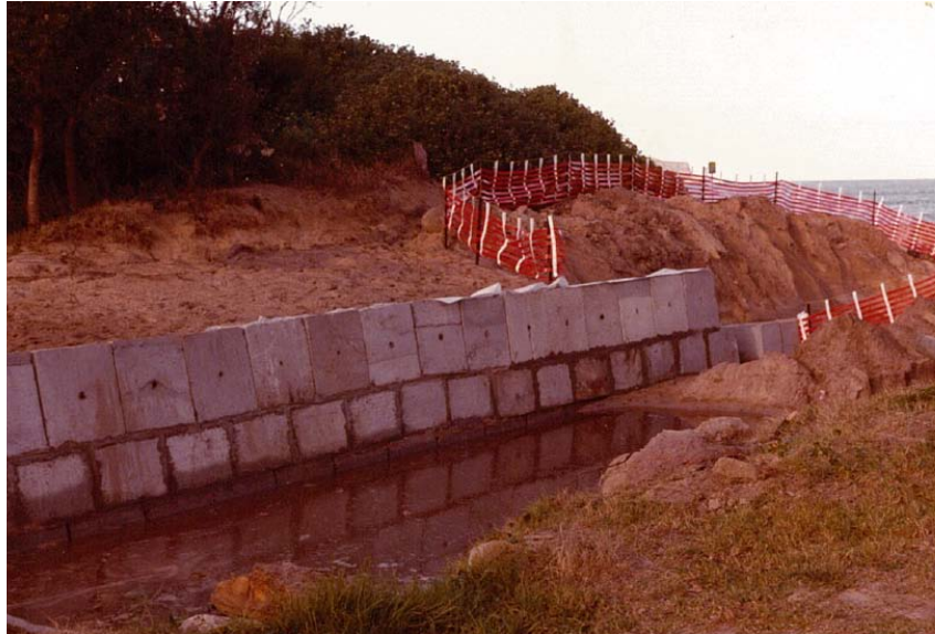
Figure 2-1 Construction of the entrance training wall at Pearl Beach Lagoon (Source Peter Bayliss)
