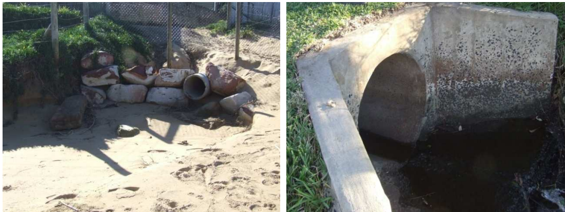
Stormwater outlets at Avoca (left) and Cockrone Lagoon (right)
