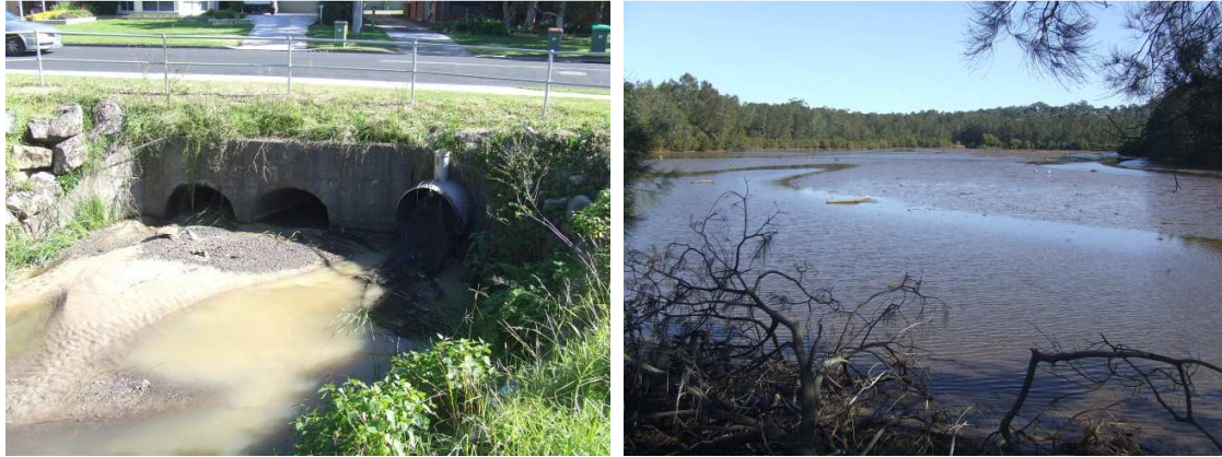
Stormwater input resulting in sedimentation at Wamberal (left) and Terrigal Lagoon (right)
