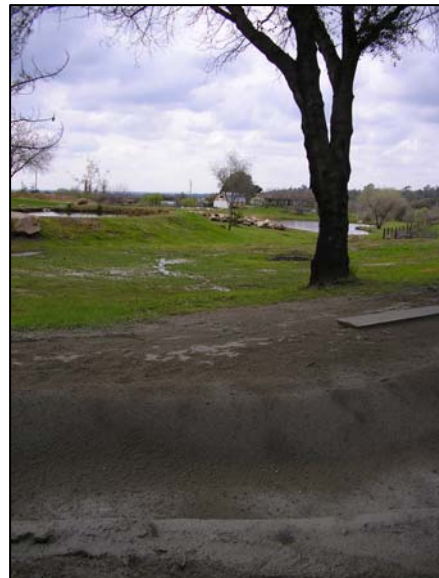
Ponding on landowner property due to seepage visible in background, and recent lining on Baughman Canal
