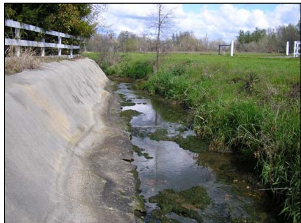
Algae growth within Boardman Canal downstream of Mammoth Reservoir
