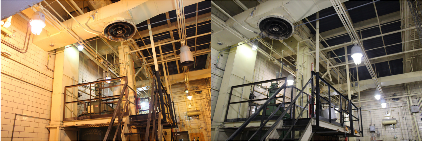
Before: 250W High Pressure Sodium Lamps
