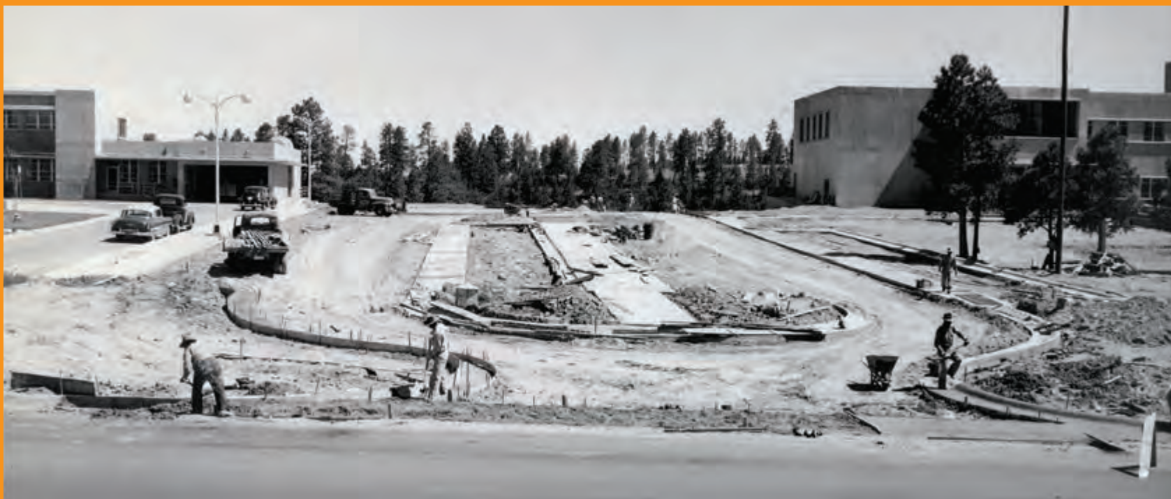
The Health Research Laboratory under construction on the right, with the Los Alamos Hospital (present-day Los Alamos Medical Center) on the left, June 15, 1953.
