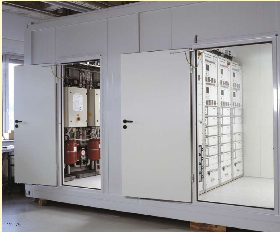
FIG 1 State-of-the-art container transmitter with eight 800 W DVB transmitters.
