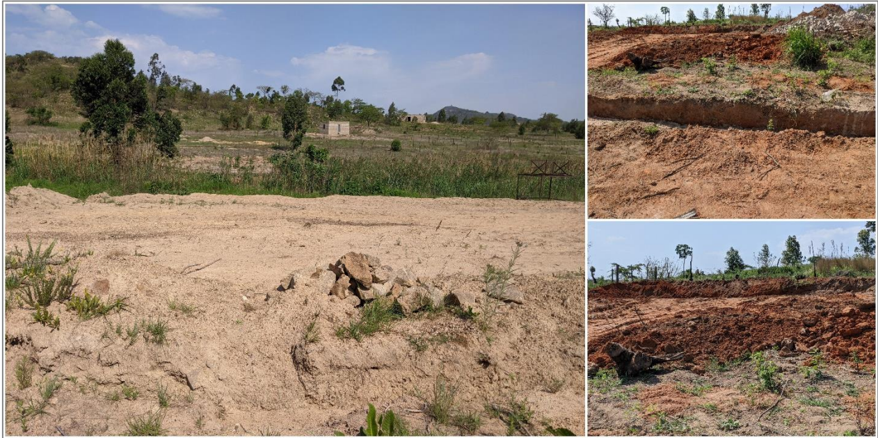
Figure 3 Transformed state of the proposed site with household plots being cleared along the site footprint
