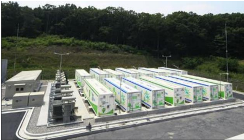
Figure 4-3: Example of a Lithium-Ion BESS installation
