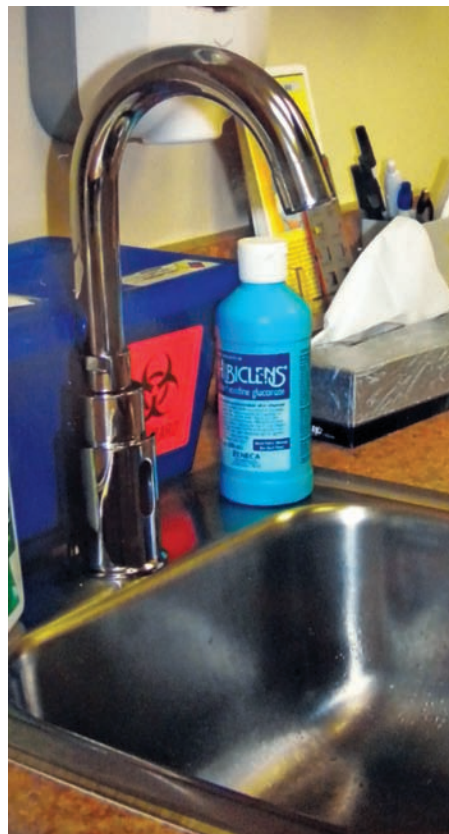
Sink prior to electro-desiccator use.
