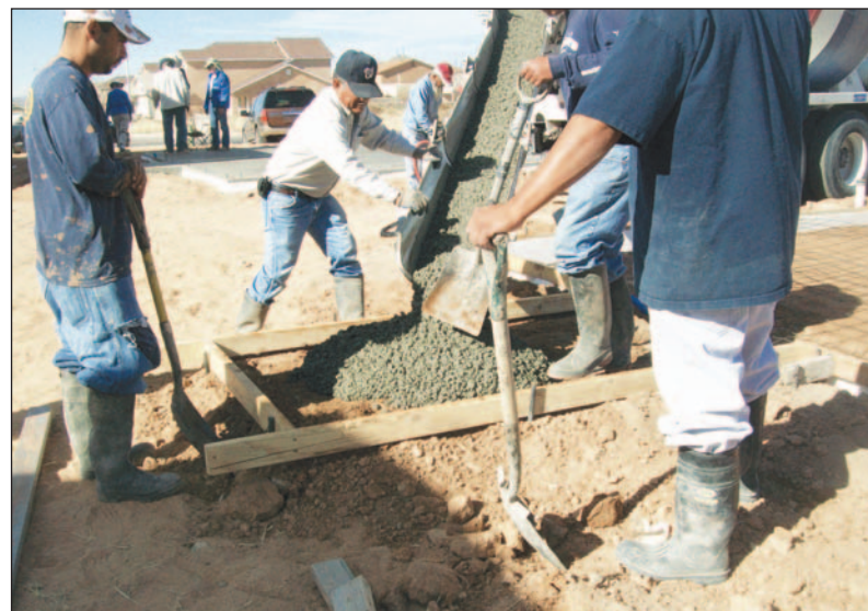
The layout of the four-bedroom home on Calle Bella built by Mesilla Valley Habitat for Humanity before the concrete is poured Tuesday, Dec. 14.
