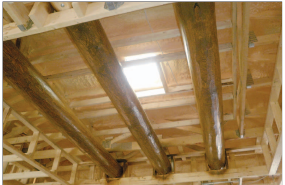
Now in the framing stages, the new home built by Clifford in the Pueblos at Alameda Ranch is being constructed to include green and energy-efficient techniques and materials, including spray foam insulation.
