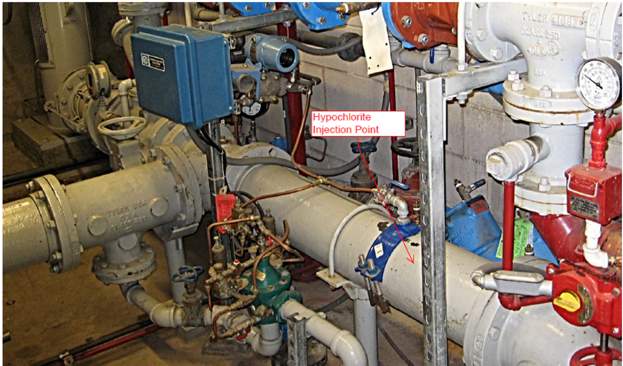
Figure 5-20. Hypochlorite Injection Point
