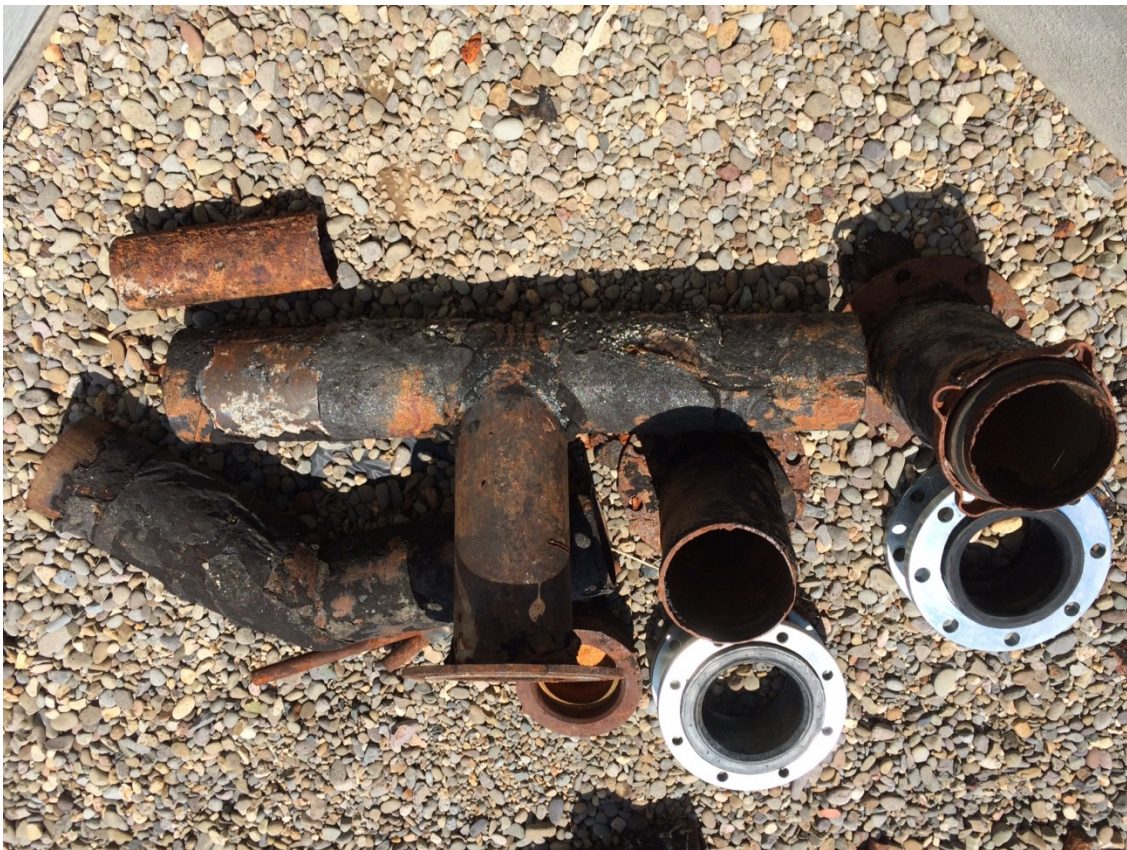
Photo 3-6. Failed Pipe Examples
