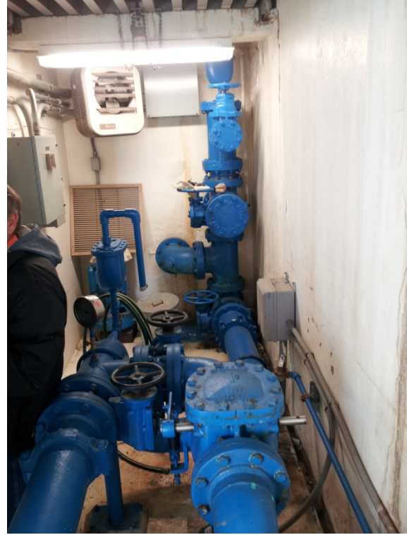
Photo 3-5. MBPS Discharge Piping
