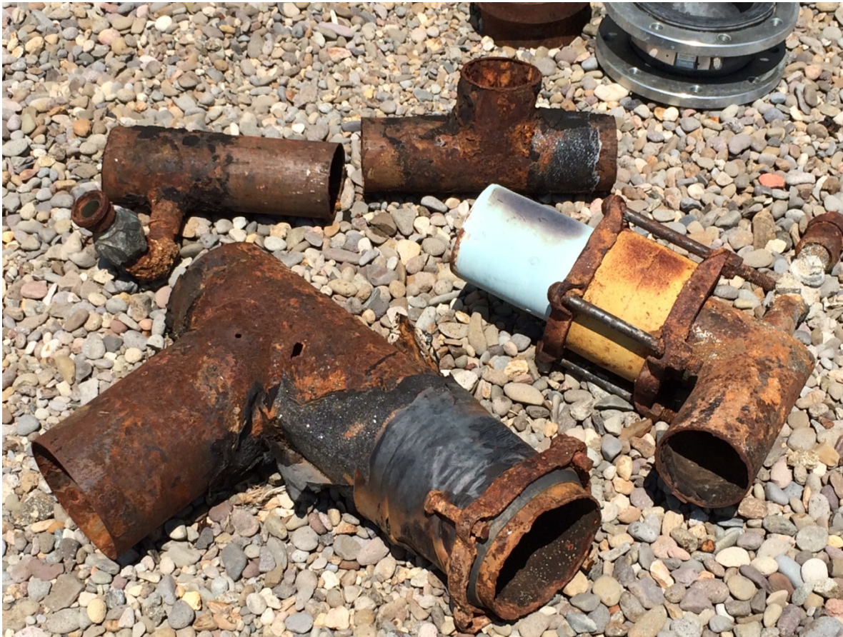
Photo 3-7. Typical Failed Pipes
