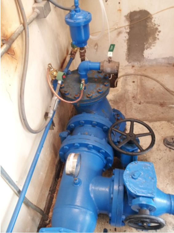
Photo 3-4. MBPS Intake Piping
