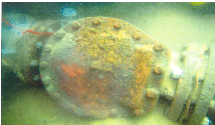
Photo 3-3. Original Tilted Check Valve
