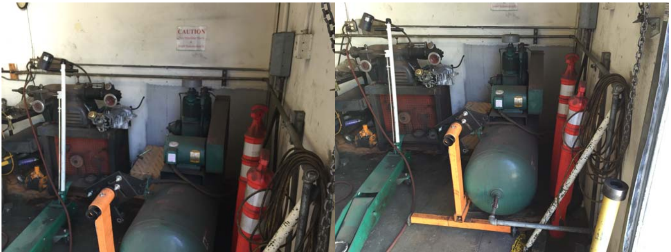
Discount Tire Center Lake Forest Air Compressor
