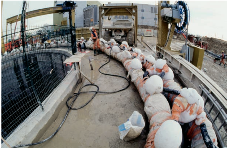
11 Freezing of ground with liquid nitrogen to overcome unforeseen ground conditions during the excavation of the CMS shaft.
