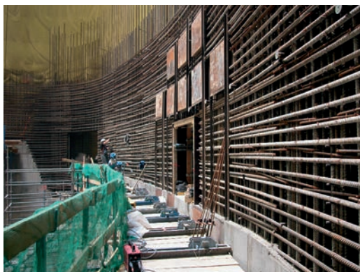
23. A view of the welded lattice reinforcement used in the CMS cavern.
