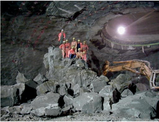
16. Excavation of ATLAS. The cavern is the largest ever built in the type of rock encountered in the Geneva basin.
