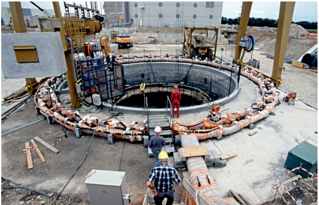
20. An underground river made the excavation of the shaft of the CMS cavern very difficult. A ring of pipes carrying liquid nitrogen was used to form a wall of ice inside which the shaft was excavated and lined with concrete.
