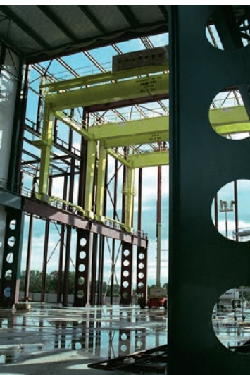
30. View of the metal frame of the SMX building under construction at the CMS construction site.
