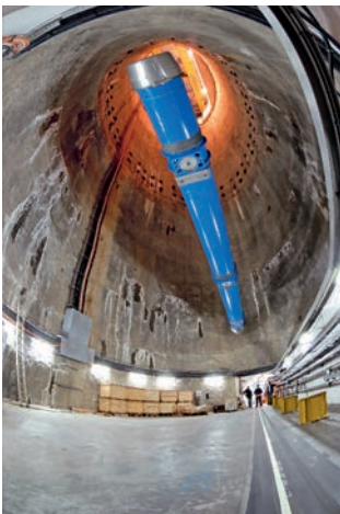
19. Image of dipole (left) being lowered into the LHC tunnel; and (right) a photo of the installed dipole with an open connection.
