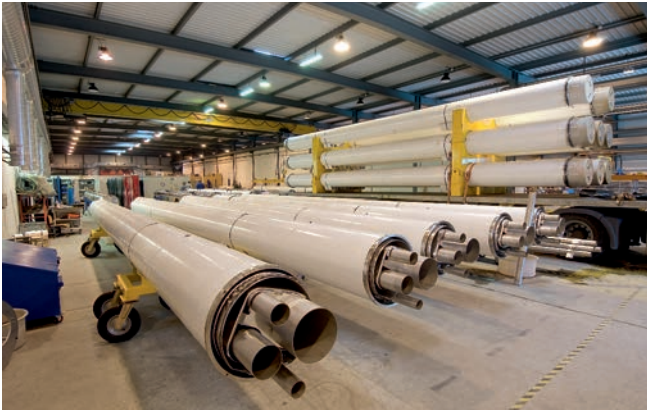
14. Dismantled sections of the cryogenic transfer line awaiting repair.
