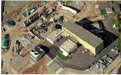
11. Aerial view of the CMS construction site, showing the building used for the construction of the yoke.
