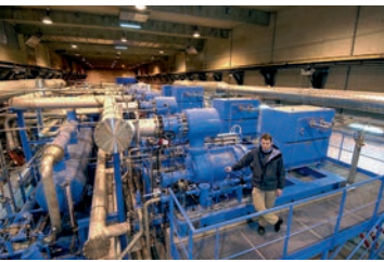
53. 4.5-K-helium refrigerator for LHC: compressor station (top); and cold boxes (middle and bottom).
