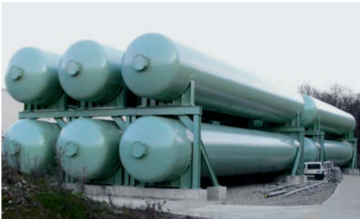
58. 250 m 3 storage vessels for gaseous helium at medium pressure (2 MPa).
