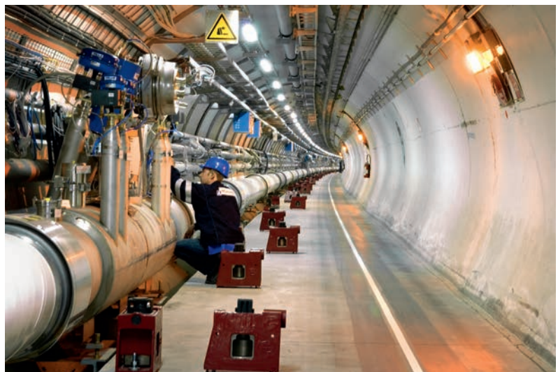
13. The 27-km cryogenic distribution line before the installation of the dipole magnets.
