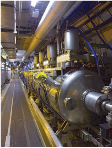
106. The RF modules after final installation in the tunnel.
