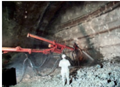
20. A view of the use of hydraulic rock-breakers during the construction of the ATLAS cavern.
