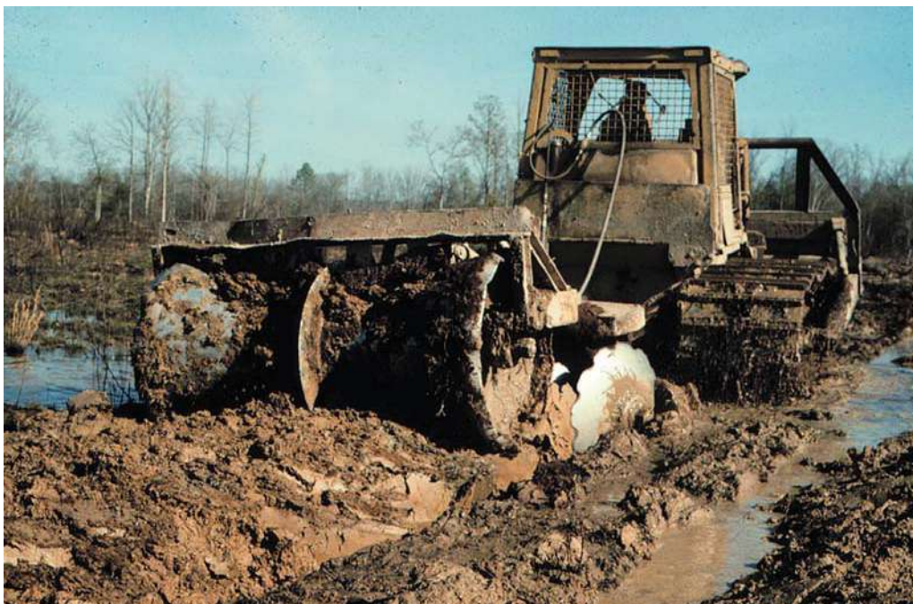
Figure 23.10 —Bedding as a final step in site preparation prior to planting on an upper west Gulf Coastal Plain site in Bradley County, Arkansas. (USDA Forest Service photograph by James M. Guldin)
