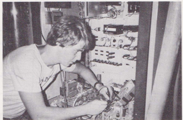
Testing on one of the controllers.
