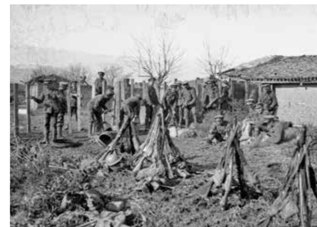
5.6 British troops constructing a street barricade in a recently captured village in the Struma Valley, autumn 1916 © IWM
