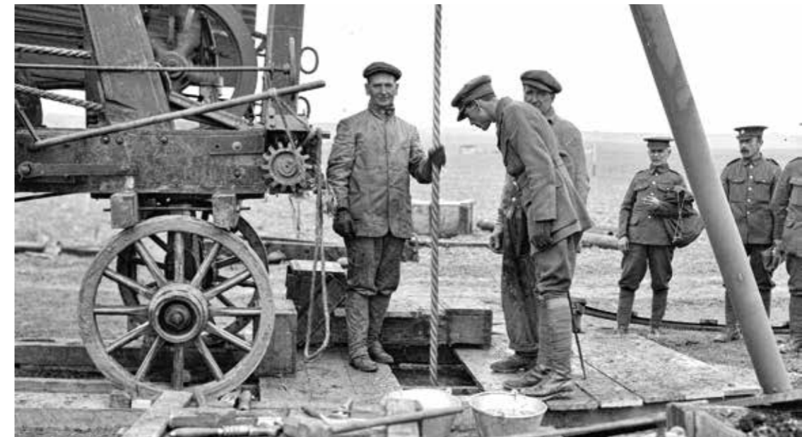
5.8 Royal Engineers boring an artesian well to supply water at an army camp near Salonika in 1916 © IWM
