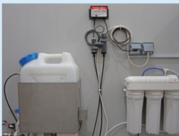
Water treatment systems
