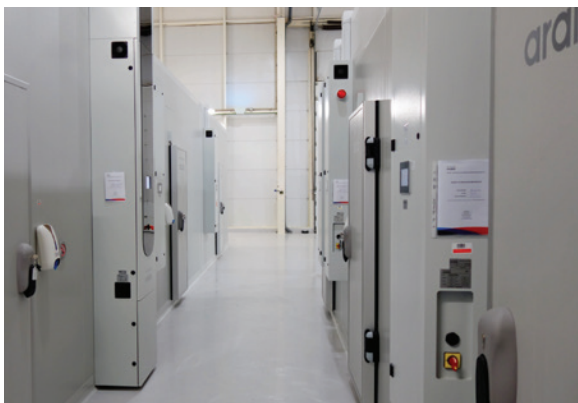
SET OF 8 X FITOCLIMA STABILITY ROOMS AT A STABILITY SERVICES COMPANY
