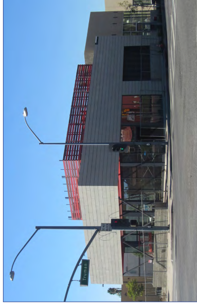
View of a new restaurant building under construction on the corner of Truman Street and Maclay Avenue.
