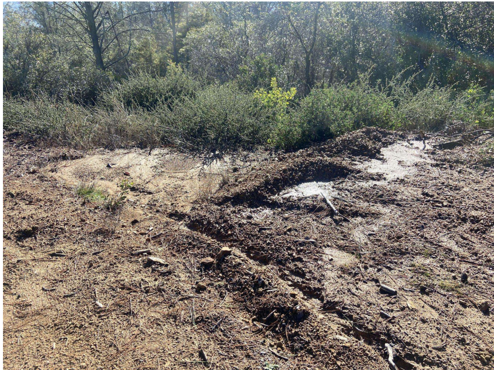
Photo 2. Location 2: Road conditions after rain.
