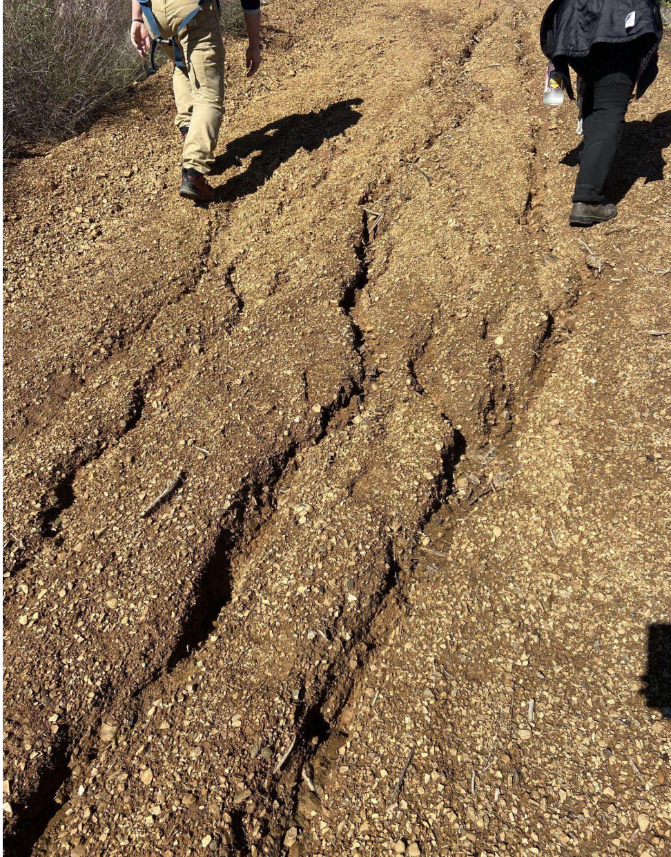
Photo 14. Location 11: Severe water damage to road.
