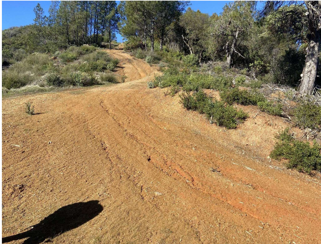
Photo 4. Location 4: Erosion on roads, walking west from Location Number 3.
