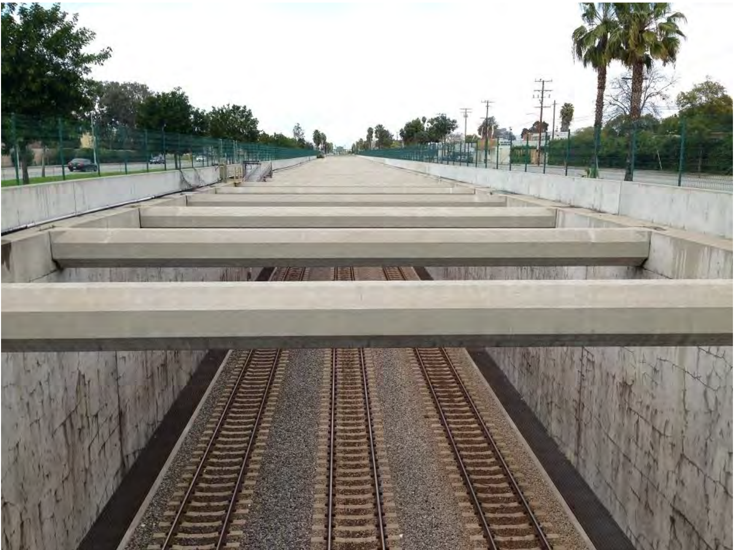
Fig. 3. A section of the Alameda Corridor's mid-corridor trench in the city of Compton. Photo by Brian Yanity
