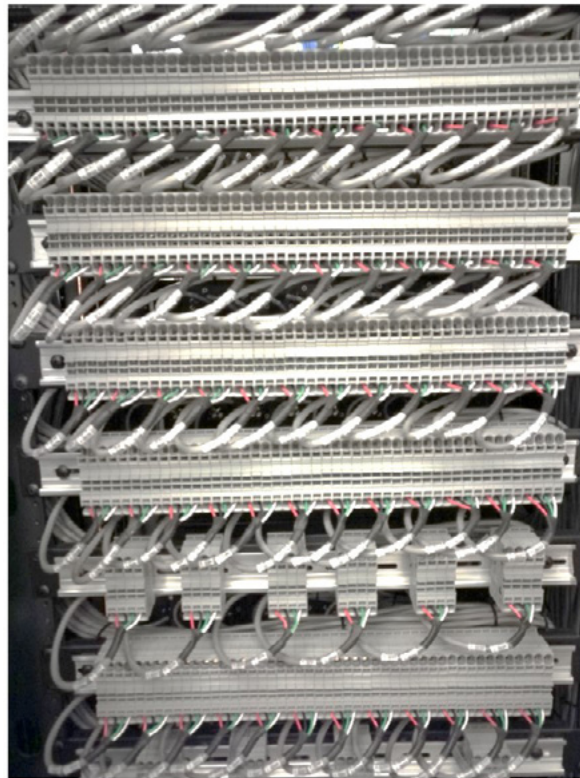
Installed Partyline Intercom Cabling that is easy to Validate and Maintain
