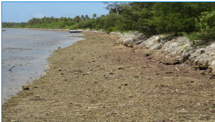
The worn out rock revetment from Kanokupolu and 'Ahou.
