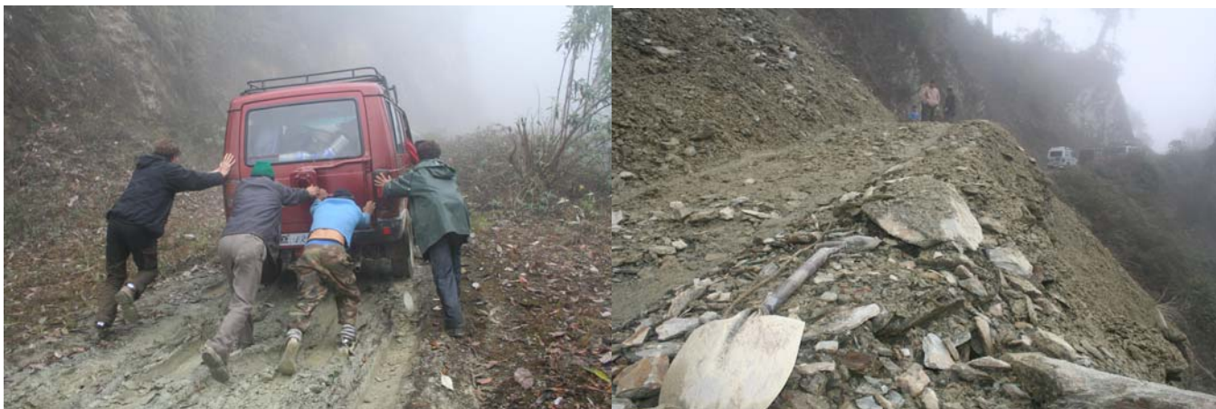
Near the pass at Eaglenest, there is a rather dangerous land-slide that almost collapses at every rain. There was however a team of intrepid workers that cleared the road for us.
