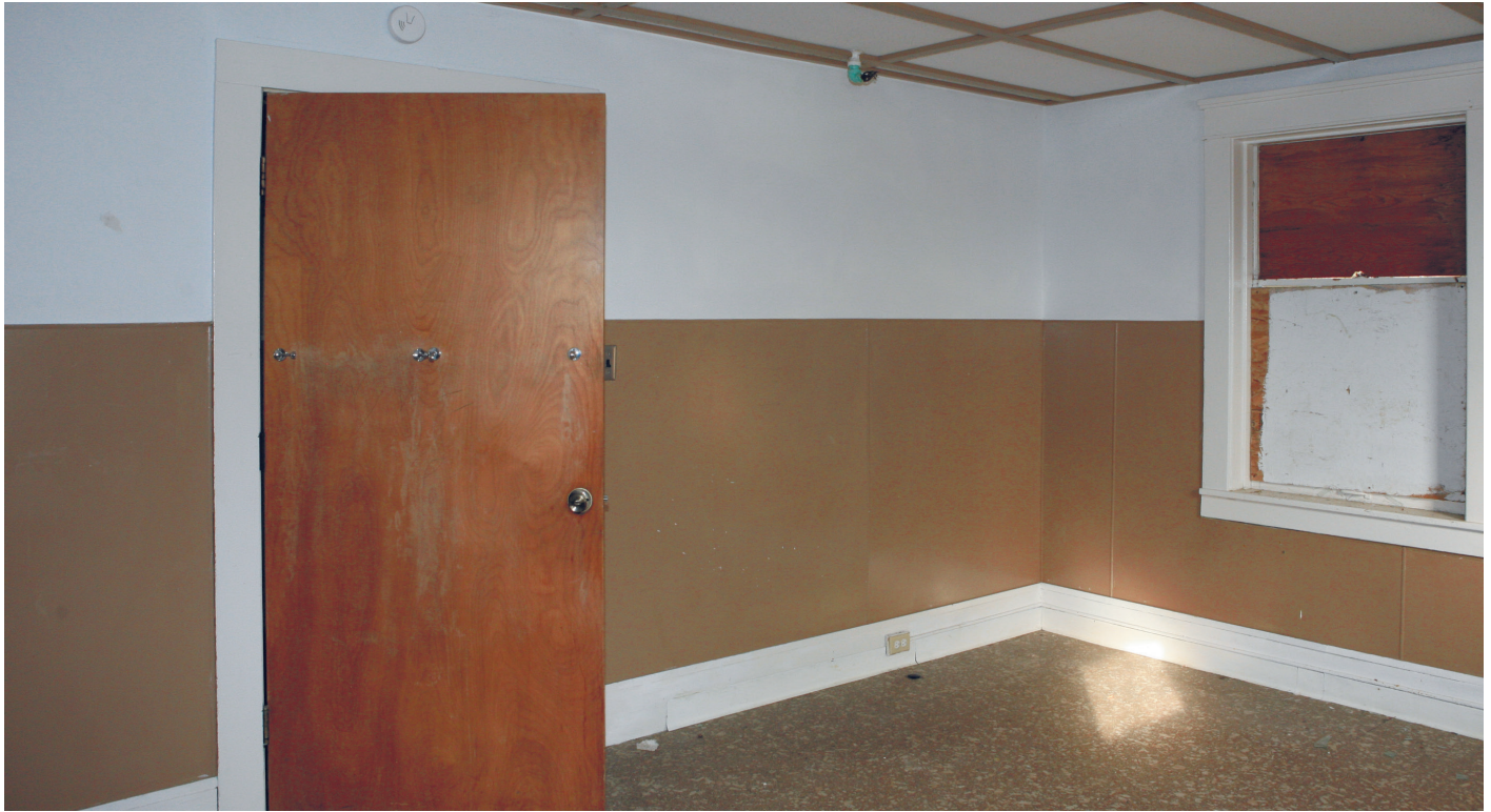
CP11. First floor, typical room. East side of main corridor. Looking NW.
