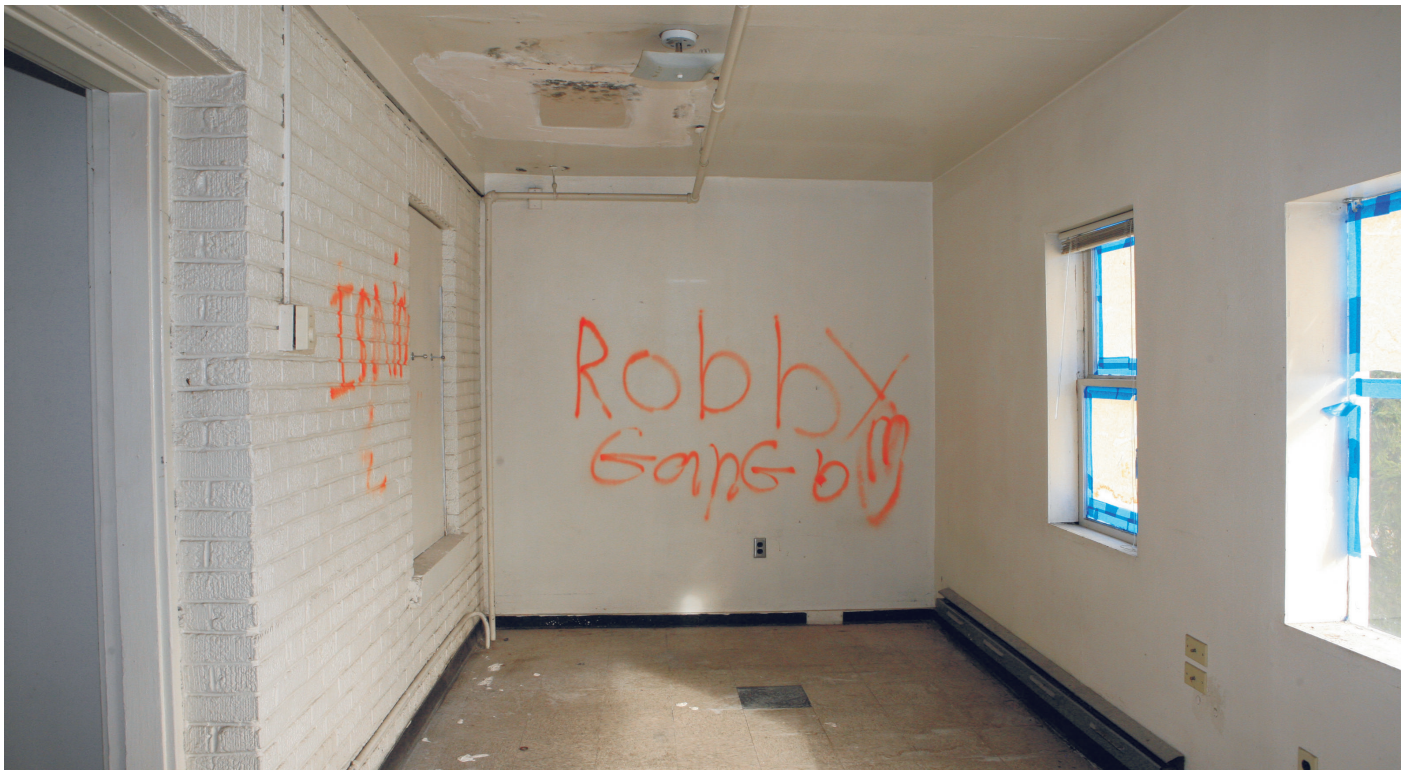
CP18. Second floor, looking north inside altered space over front (east) porch.
