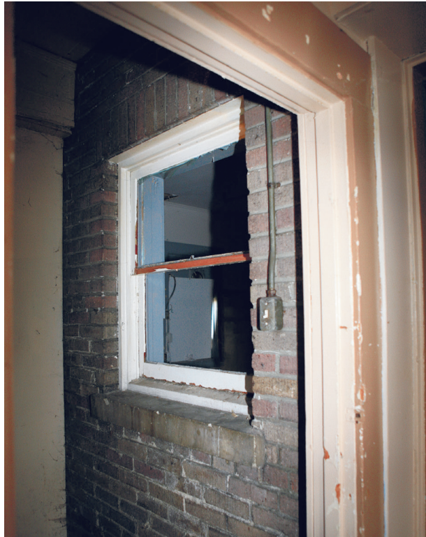
CP13. Detail of original west exterior and window; now housed within small 1-story addition, NW corner of building.
