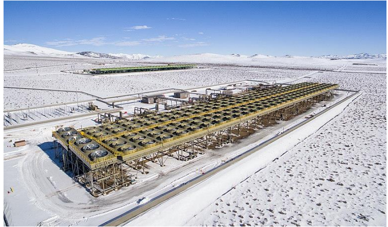
McGinness Hills Geothermal Plant | Source: Nevada BLM
