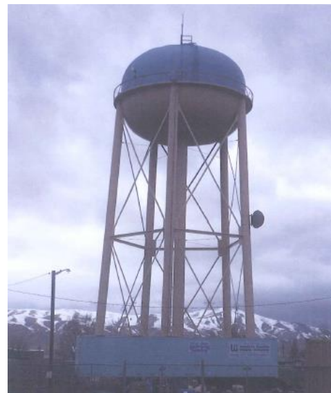
Abandoned 300,000-gallon Water Tank, to be demolished or repurposed for non-potable water
