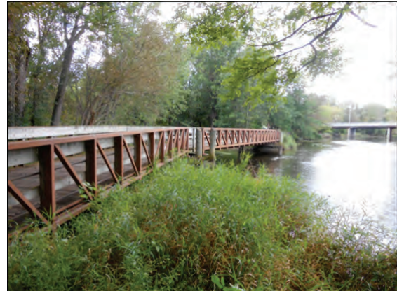
Structure: CL-18-LTE-RC City of Lansing – Bridge #18 - Lansing River Trail East - over Red Cedar Creek
