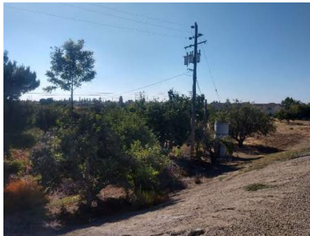
Figure 17 – View of transformers adjacent north near levy.
