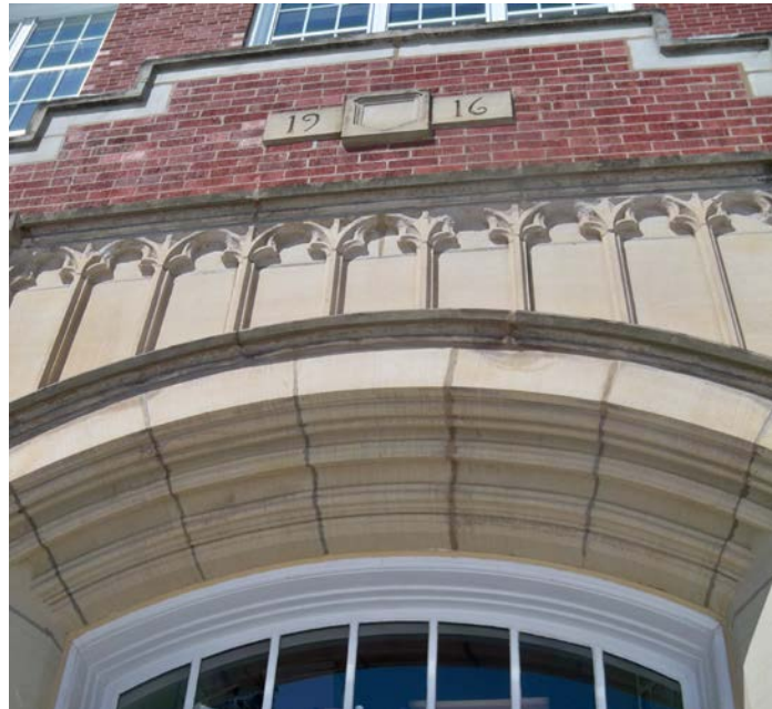
The original portion of the school, now Olmsted Falls City Hall, shows the 1916 date of its construction above one doorway.
