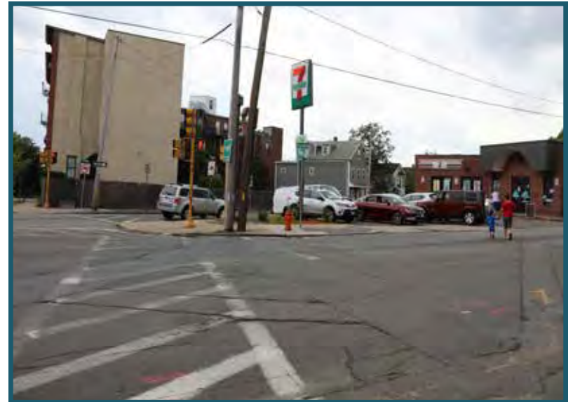
Faded pavement markings at Broadway/Tremont Street intersection
