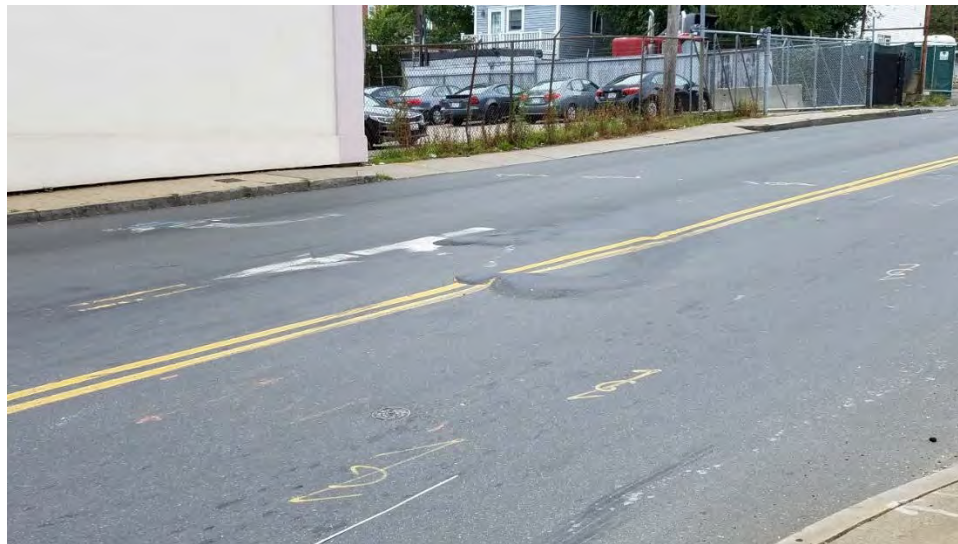
Image 2: Williams Street at Pearl Street – Williams Street approach showing worn pavement markings and rutted pavement.
