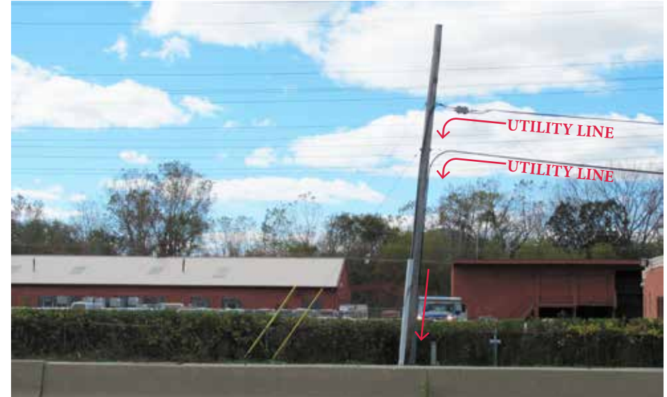
Utility Equipment Burial. Business along Highway 41 buried utility lines. Utility lines are directed underground from utility pole.
