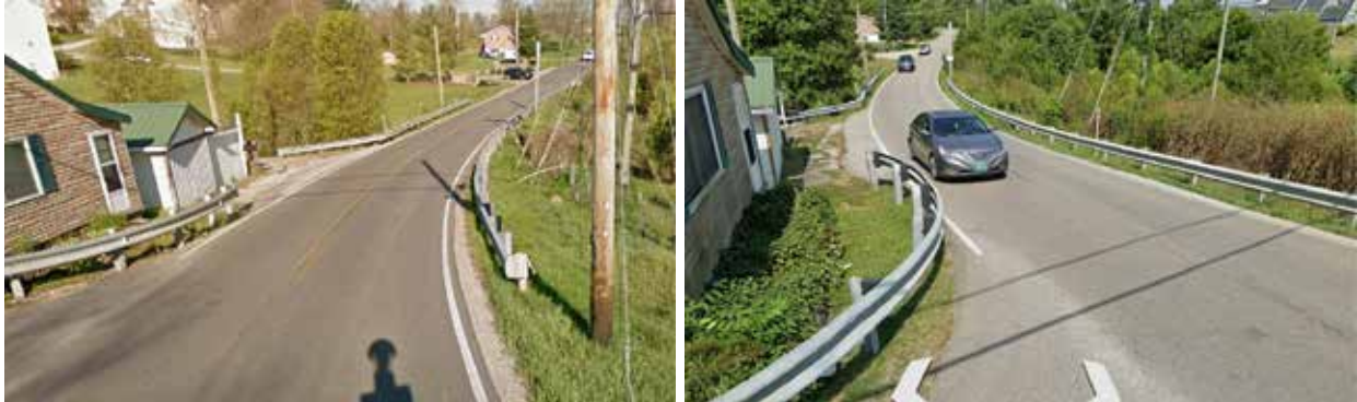
Figure A6-9: Narrowed Roadway near Richwood Church Road
