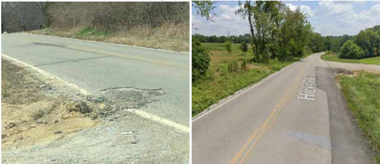
Figure A6-10: Before/After of Edge Drop off and Pothole Repairs along Hicks Pike .
