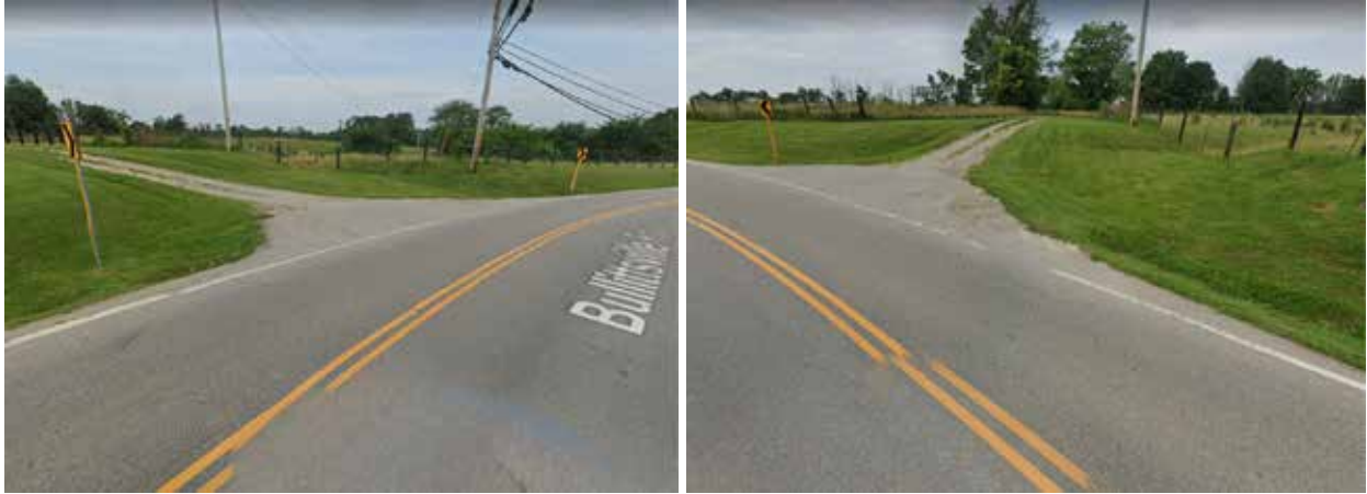
Figure A8-4: Gravel washout at Horizontal Curve
