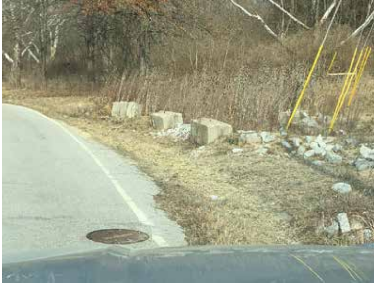
Figure A10-8: Fixed Objects east of Elijah Creek Crossing
