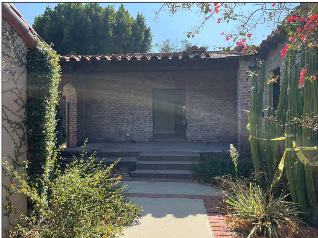
Figure 18. Overview of the concrete porch and northeast façade of the main wing, looking southwest.
