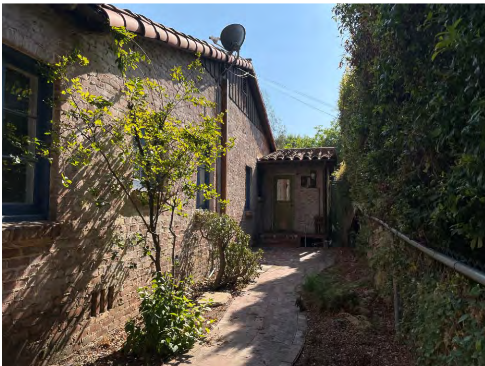
Photo 4. Overview of northwestern façade at the northern property boundary, view to the southwest.
