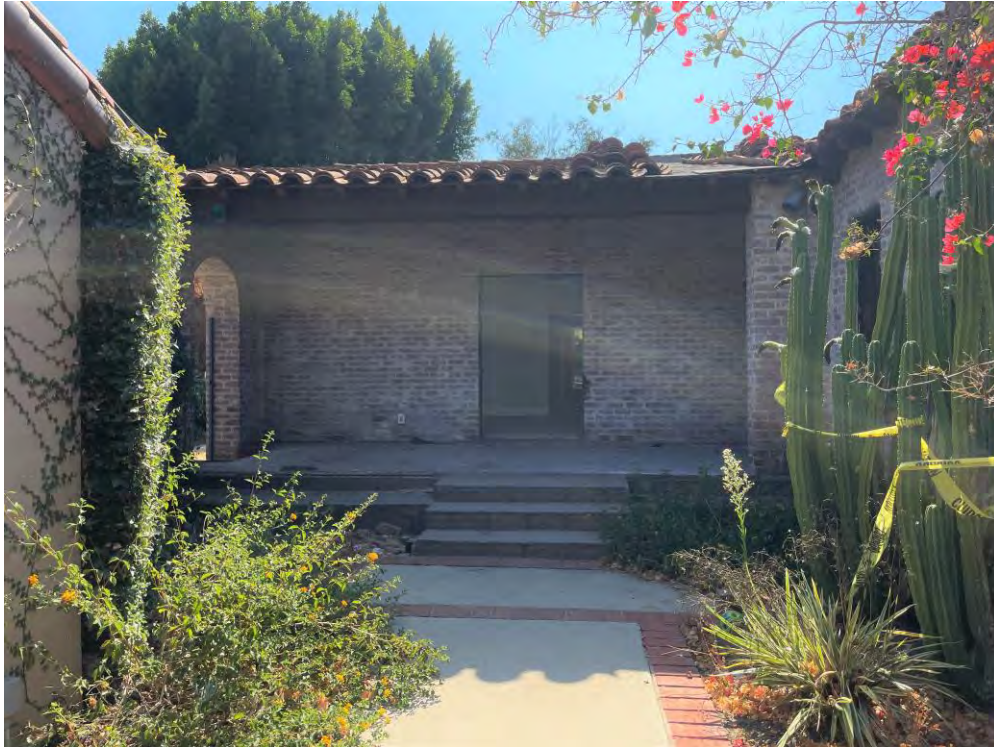
Photo 3. Overview of northeastern porch and primary entrance (door missing) on the rear east façade of the main wing, view to the southwest.
