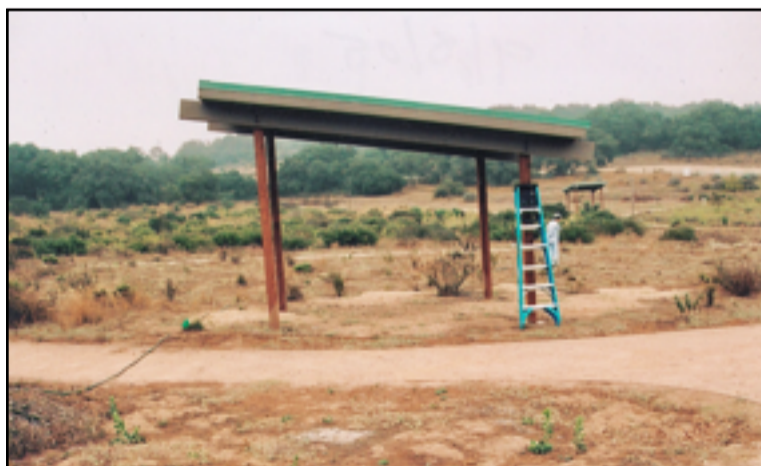
Photos: Upper Right: Installing the Riparian Domain. Below: The Kiosk installed in the late 1990s, and as it is today
