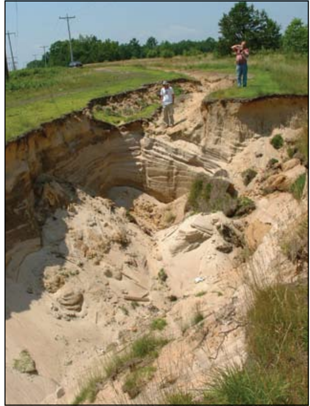
Researchers examine rapid and severe erosion on conservation land near McGuire Road, in Kennebunk, in the Branch Brook watershed. Motorized vehicles cut through the thin topsoil exposing highly erodable sand. Photo Wells NERR.
