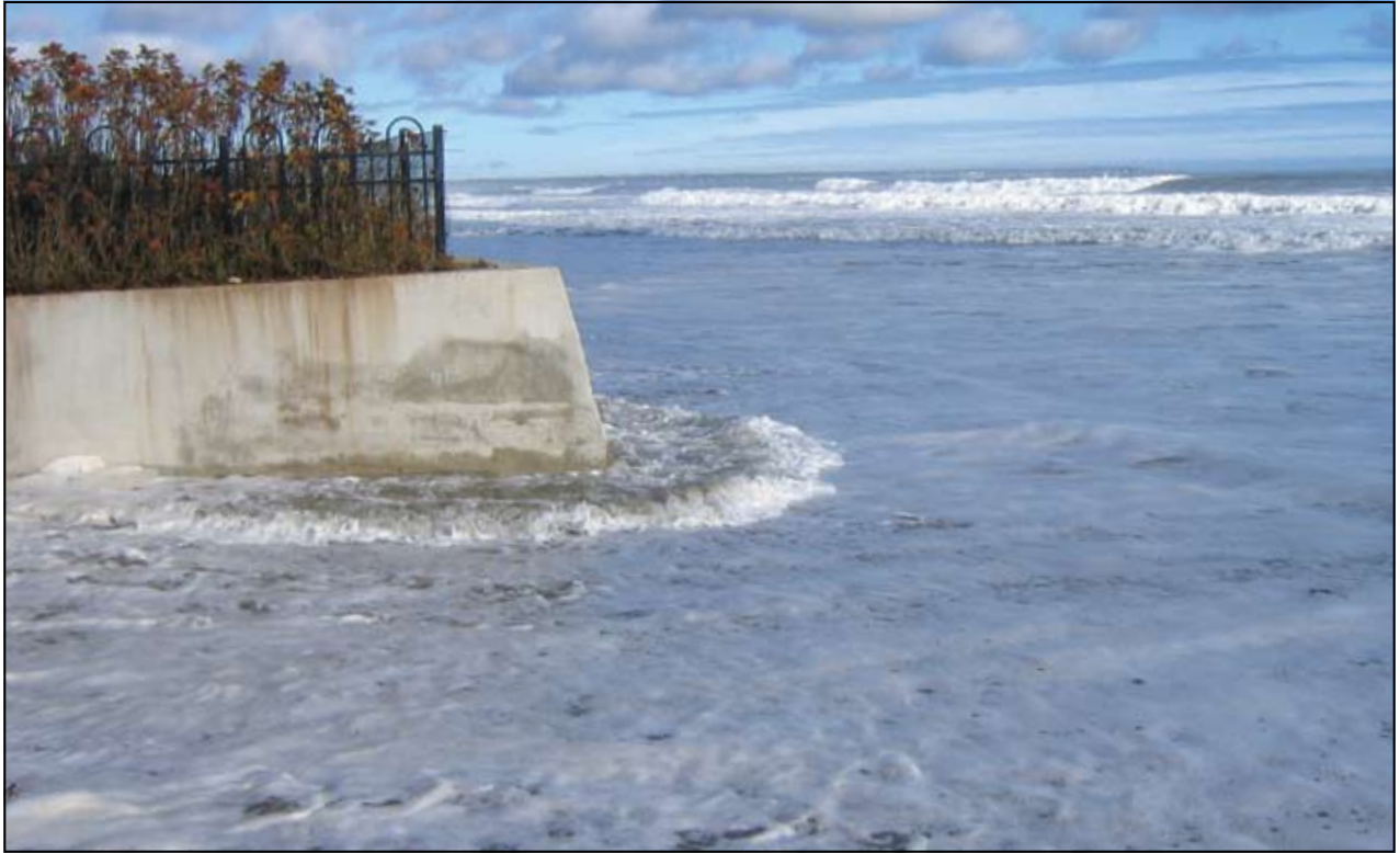
High tide at Laudholm Beach. Waves frequently reach past the ends of the concrete seawall. Photo Erno Bonebakker.
