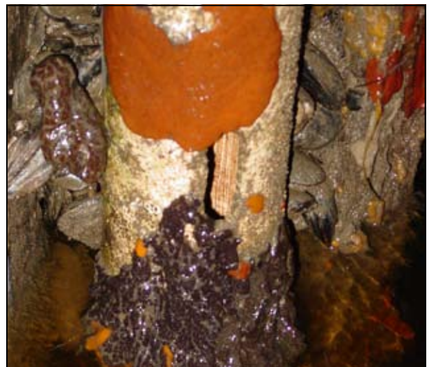
Fouling of a deployment tube for a data logger, exposed at an extreme low tide. Photo James Dochtermann.
