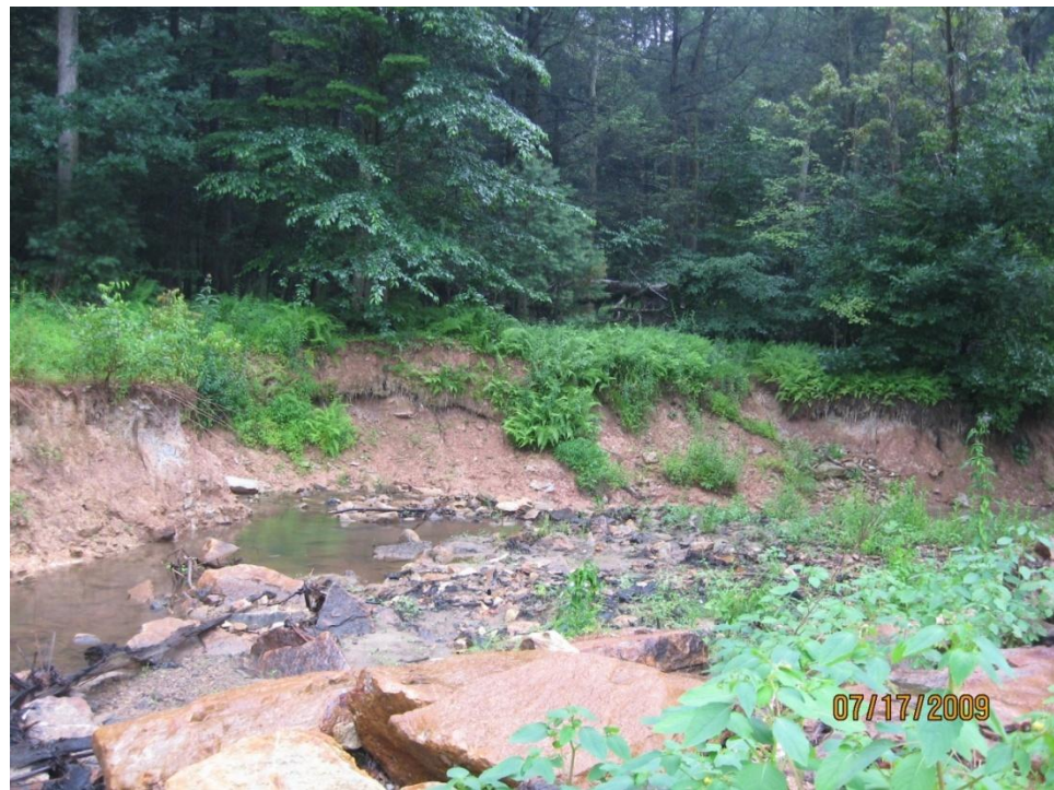
Photo 11. Breach in former emergency spillway at Burn Cabins Grist Mill leads to excessive erosion - Bank approx. 9 ft. high
