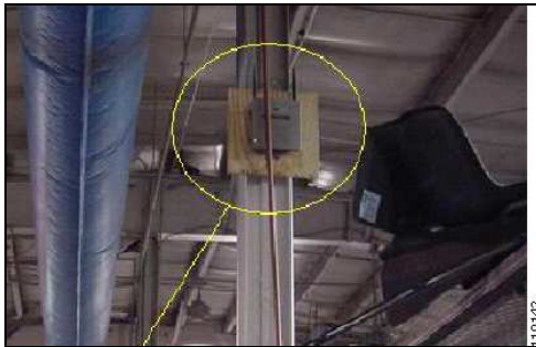
Figure D-1 Improper Placement of Antennas Near an I-Beam
