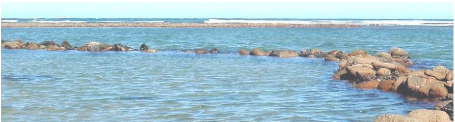
Top of fish trap wall requiring maintenance. Wave damage on waterline
