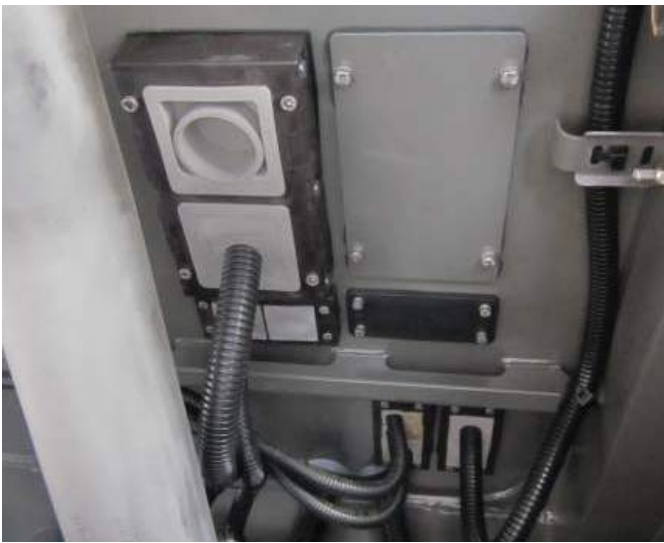
KEL-JUMBO 2 - Page 36 / KEL 24|x - Page 18 Routing of conduits and large cables between vehicle body and chassis
