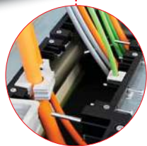
Routing of pre-terminated cables of up to 35 mm in diameter (KEL 24)
