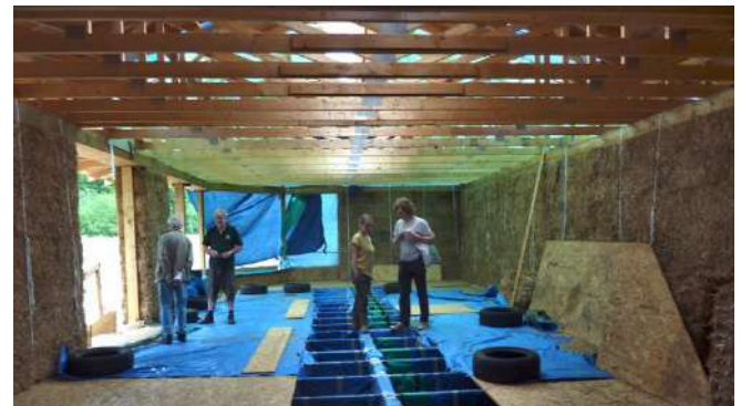
figure 2: Andy Pedley, Selborne Society Secretary, showing visitors around the new straw bale education centre now under construction at Perivale Wood.
