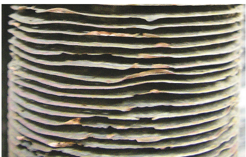
Preheater Fins After Cleaning with NitroLance
