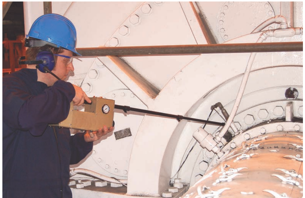
Conco Technician with SF 6 Pack Unit Checking for Sources of Air In-leakage
