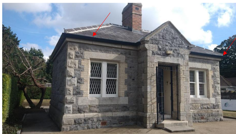
Small gaps here would allow bat access
