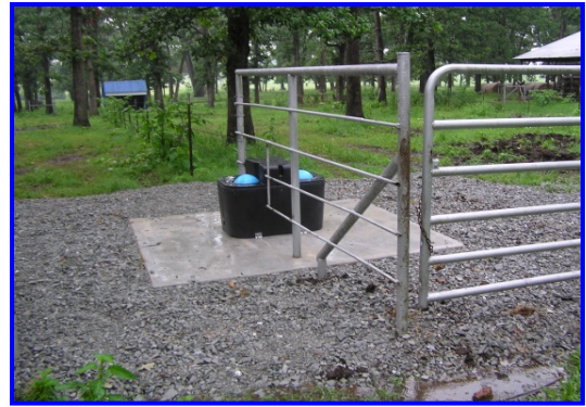
Figure 17. Alternative water supply.
