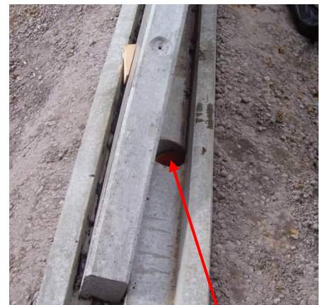
Seating Channel with Drain outlet
