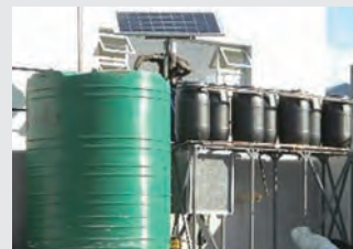
Recycling of wastewater and rainwater at some dealers
