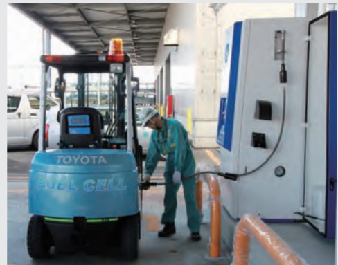
Small-scale high-pressure hydrogen gas station (Photo provided courtesy of New Kansai International Airport Co., Ltd.)
