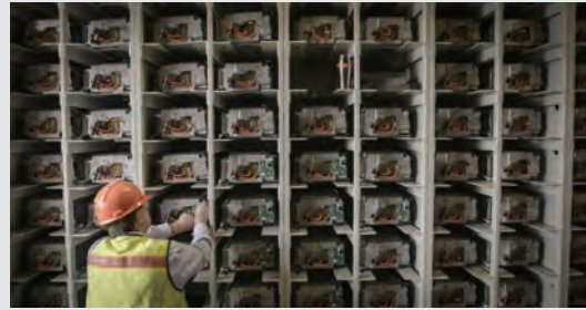
Reclaimed Camry Hybrid nickel-metal hydride battery packs
