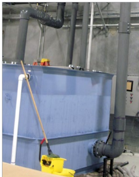
Return pipe attached at factory-installed low point connection.
