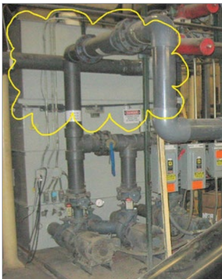
Tank with height extended to increase pump suction head (yellow cloud).
