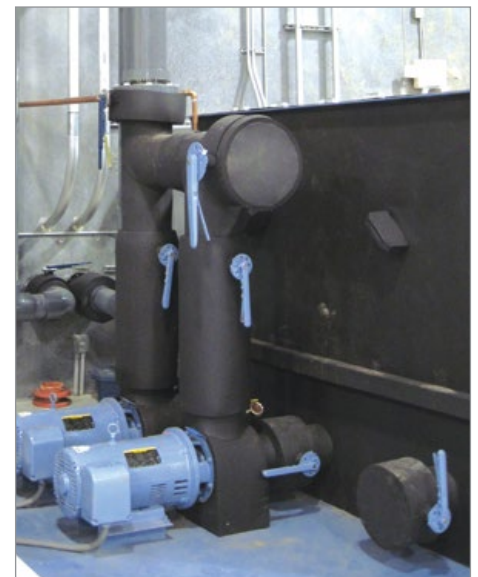
Future pump connection on tank at installation.
