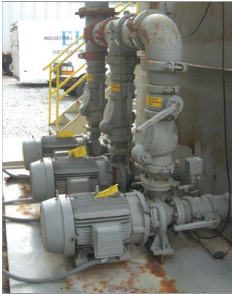
Original tank system (one pump out for service).
