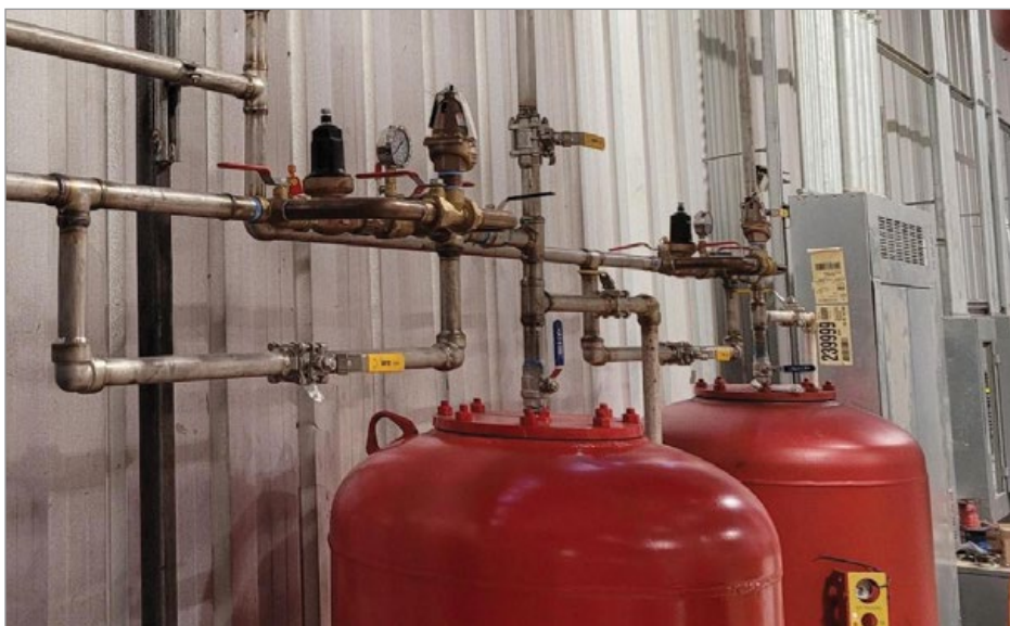
Make-up water valves and expansion tanks for two separate closed systems.
