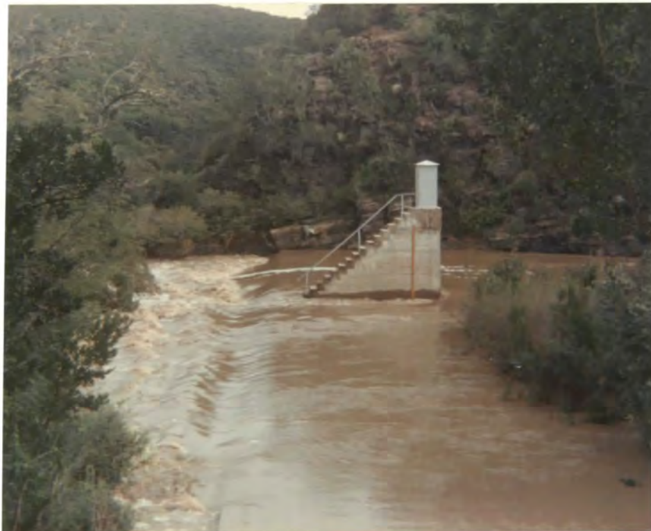
Figure 83 . Wolfcrag gauging weir on the Kowie River during high flood conditions. The gauging notch against rock-face is completely submerged.
