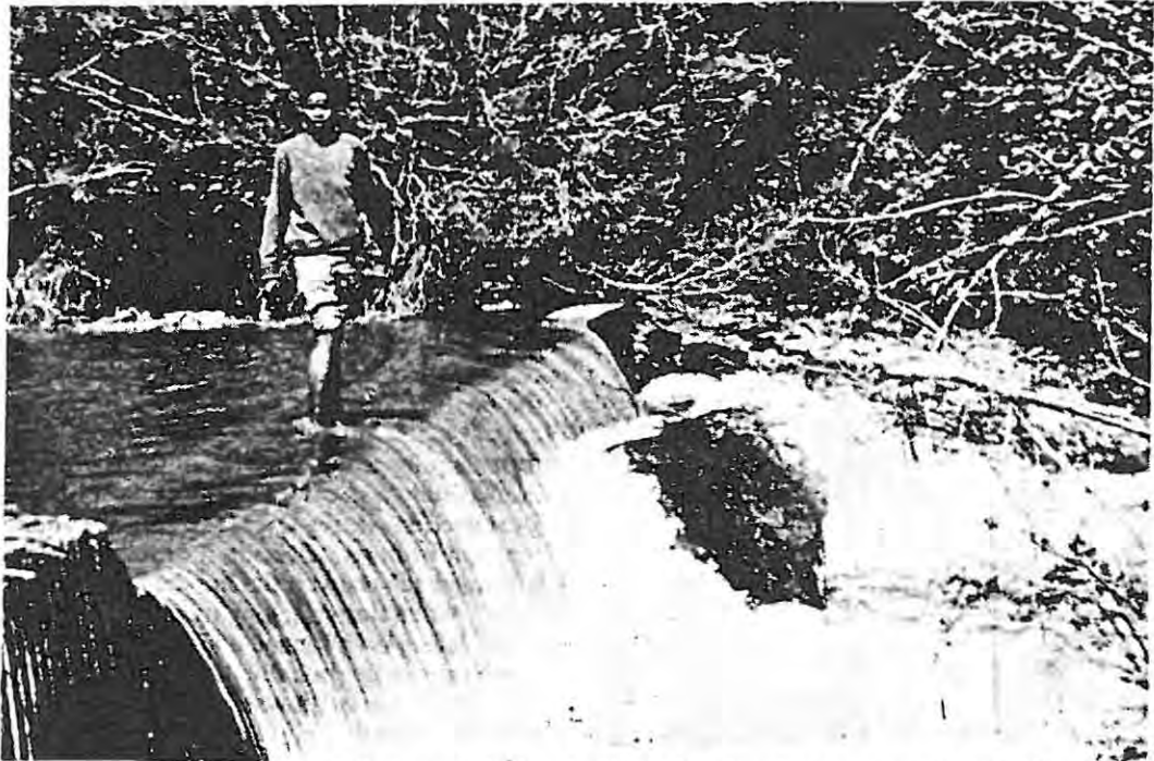
Weir on the Bloukrans River (tributary of the Kowie River), 40 kilometres upstream of the Ebb and Flow, found blocking upstream migration of mullet.
