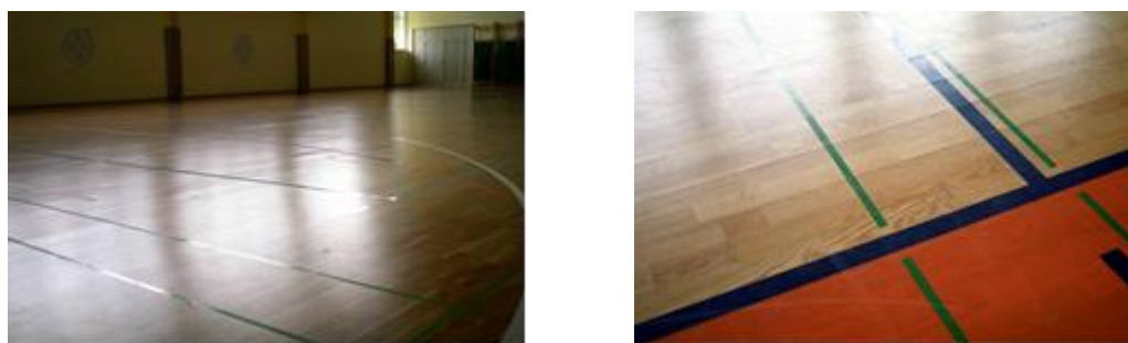
Figure 6. Uneven surface due to the moisture related movement.
