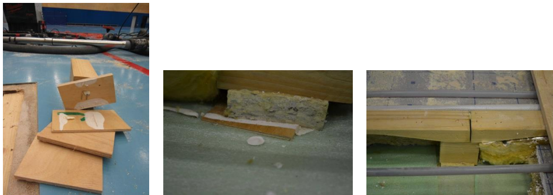
Figure 5. Poor instalation details
