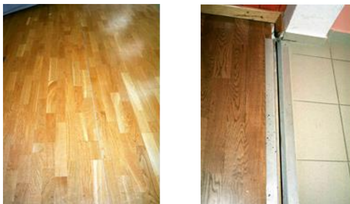
Figure 7. Cracks between parquet boards / panels with extensive voids at entrance / joints.
